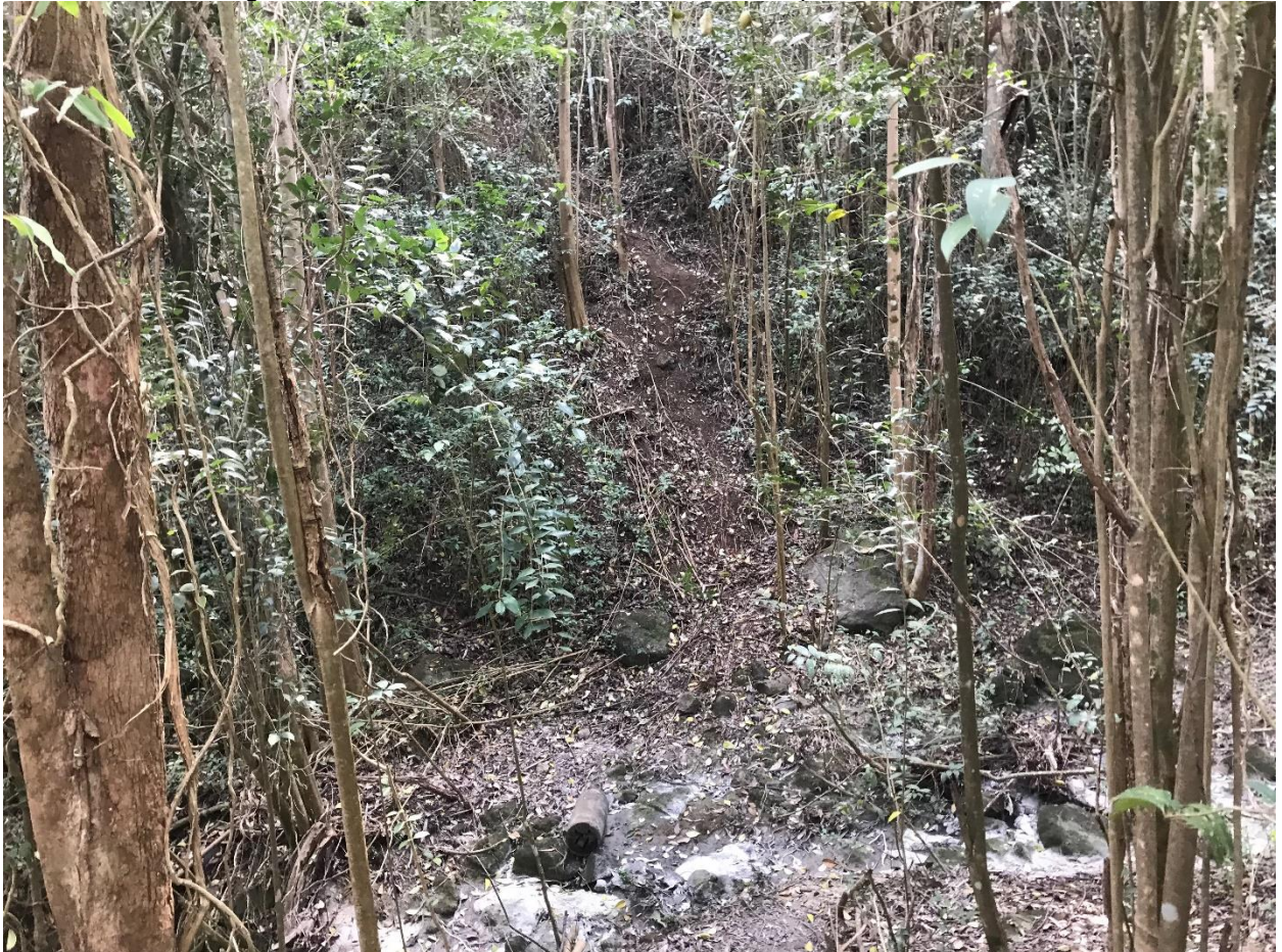
PP04 – MZ1 – Looking north from up slope. Unstable soils within impact area.
