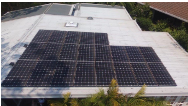
Figure 13: Typical Residential Solar PV Installation in the Shire (Source: Johnson, D, 2020)
