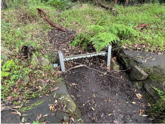
Figure 11: Full gross pollutant trap below Britannia Street
