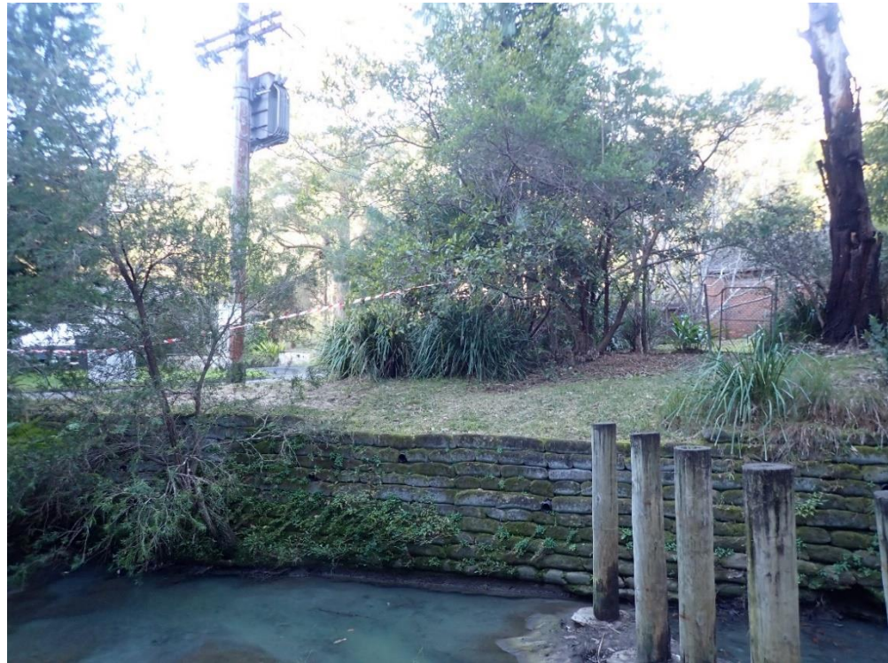
Figure 16 Exclusion tape, signage and discoloration of the water indicate sewer overflows
