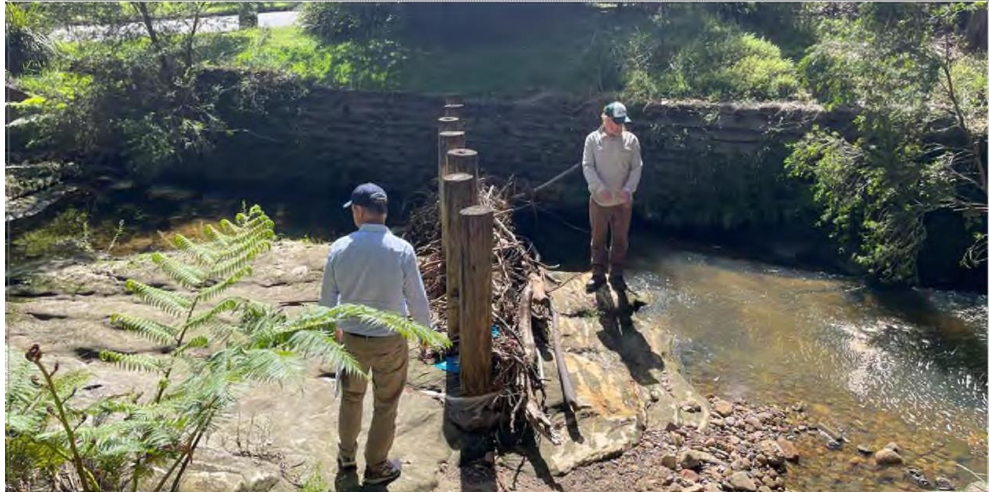
Figure 12 A row of wooden poles across the creek bed acts as a large woody debris trap
