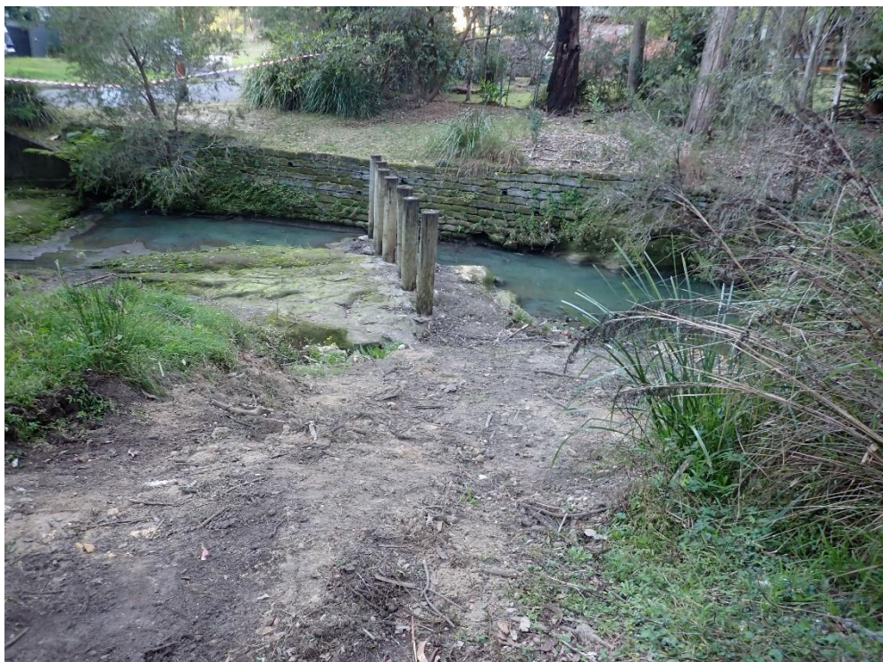
Figure 13 The woody debris is cleared from the western bank via an access point near the sewer pit
