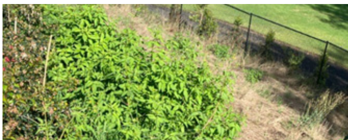
Figure 1: Weed infestation and poor growth of the eco-blanket along the western part of the northern batter along with erosion potential along the steep embankment.
