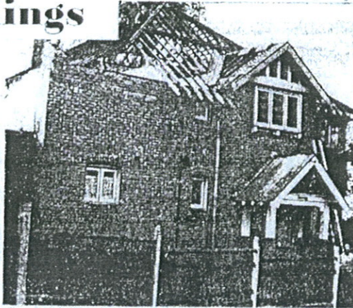
Figure 4.21 Demolition of Lyndley, 1961. Formerly the home of the Sergeant family in Hannah Street.
