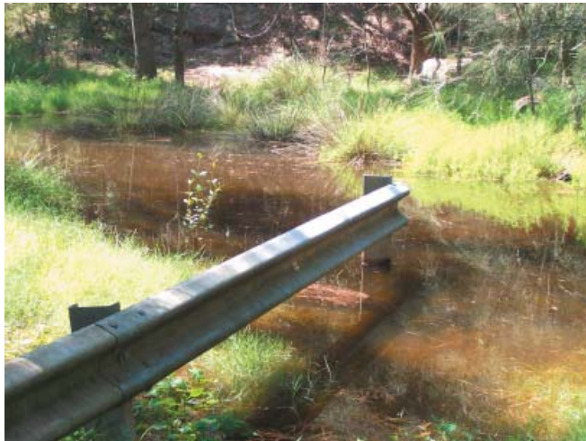
Figure 1.9: Guardrail at the northern end of the carpark flooded by a king tide
