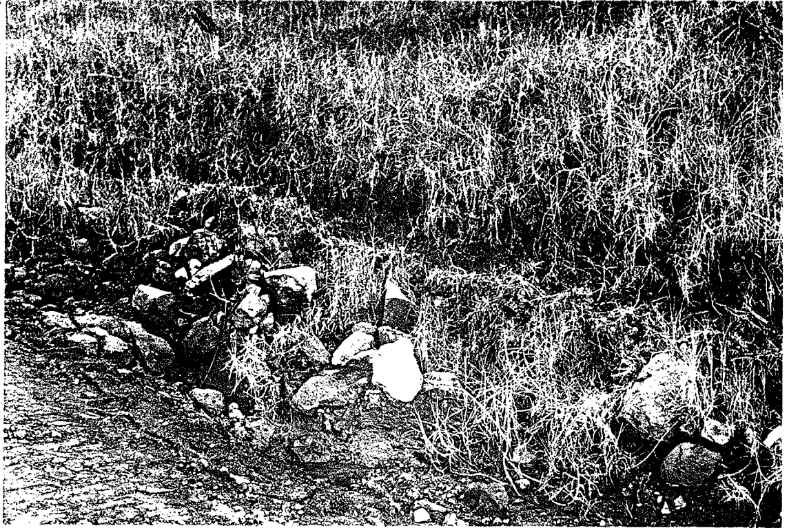
Photograph 1a - Natural drainage gully developed at (Approx. Ch.260m) boundary between northern toe of playing fields and access road. Note residual red-brown clay exposed in gully. Water in gully is almost entirely derived from seepage from toe of fill embankment.
